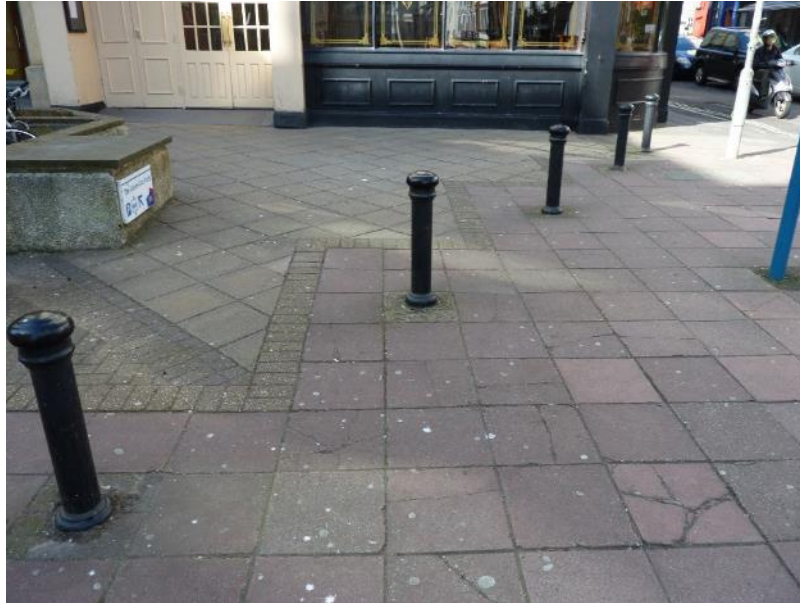
Bartholomew Square: incoherent street surfaces poorly maintained
